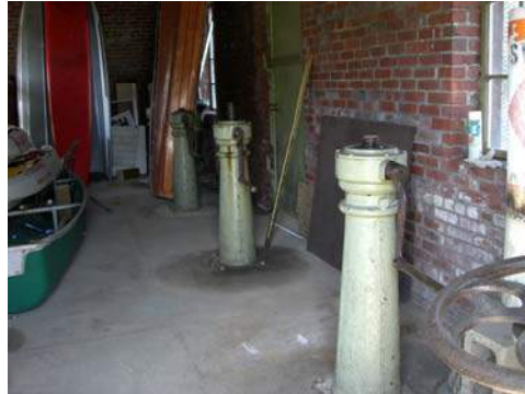
Hand cranks control sluice gates and fountain
