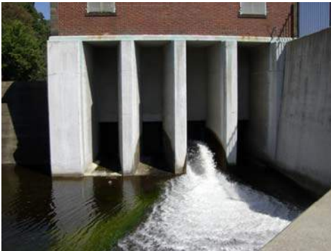
Lake Hopatcong sluice gates
